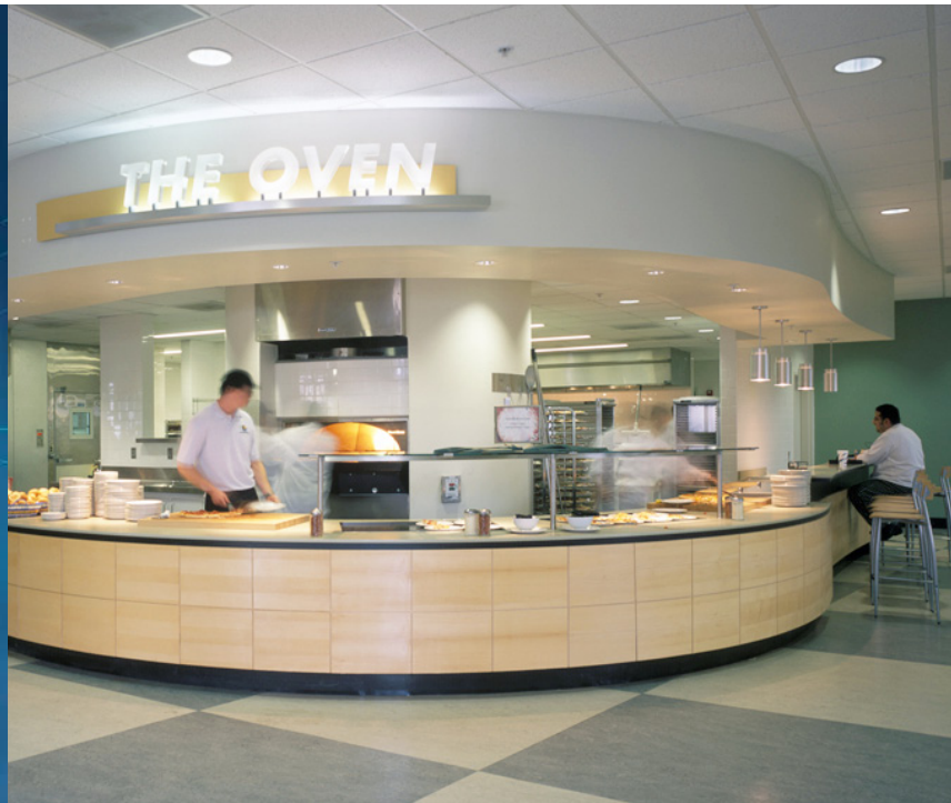
Demand ventilation fan speed controller installed at the kitchen of the Carrillo Dining Commons, University of California, Santa Barbara
