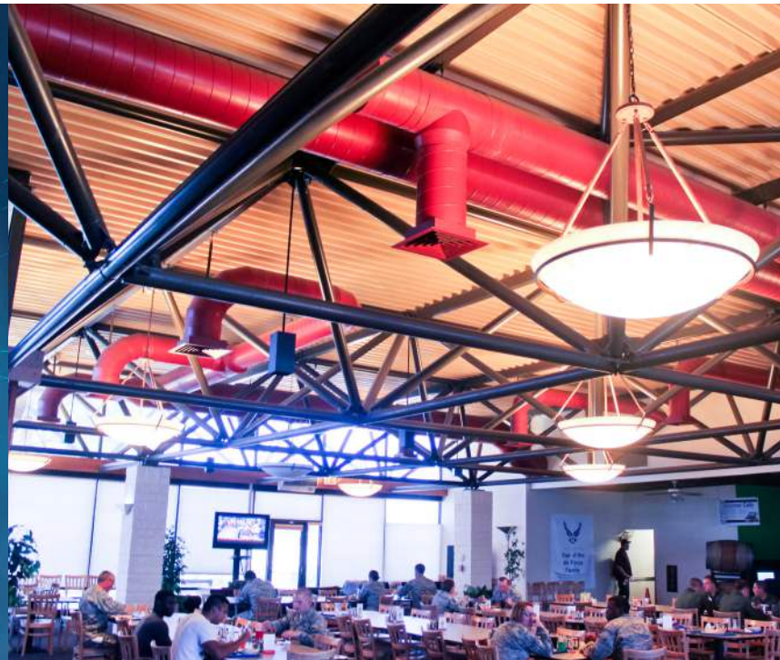
Evaporcooler condenser air pre-cooler retrofit for air-cooled chillers installed at Contrails Dining Facility at Beale Air Force Base in Marysville, California
