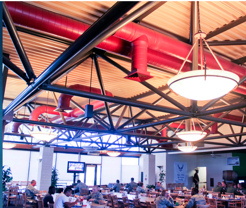
Evaporcool condenser air pre-cooler retrofit for air-cooled chillers installed at Contrails Dining Facility at Beale Air Force Base in Marysville, California
