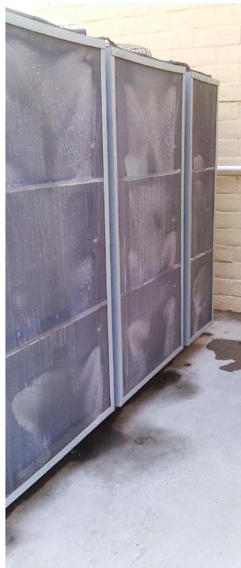
Evaporcool™ condenser air pre-coolers installed on the 50-ton Trane® Chiller at Beale Air Force Base
