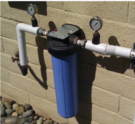
Plumbing with filtration
