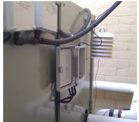
Setup of sensors and controls
