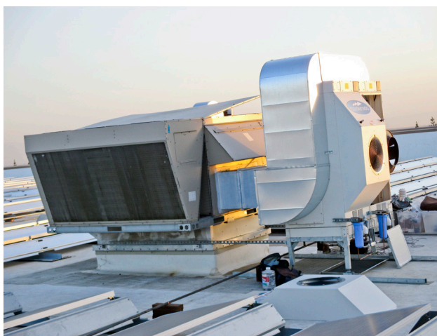
Indirect evaporative retrofit for RTUs
