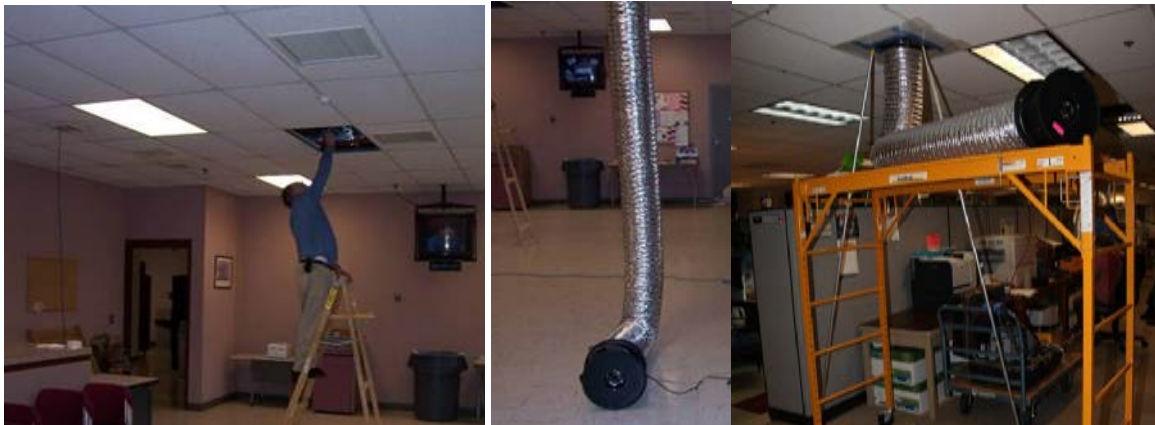
Figure 1: Example field application of modified fan pressurization protocol. VAV box inlet damper is being closed manually on the left, and the pressurization fan with integrated flow meter is attached to a supply diffuser two different ways in the two pictures on the right.
