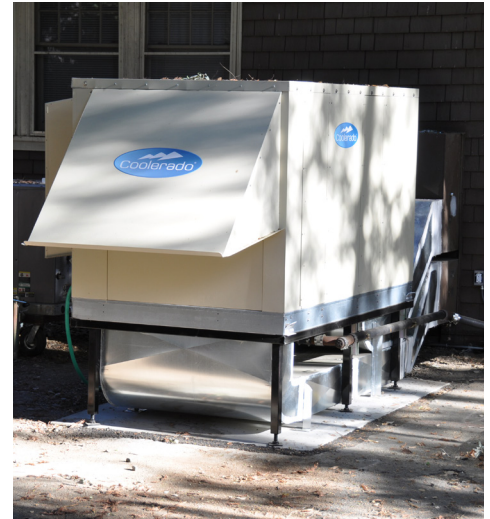
Coolerado H80 installed at the University House at UC Davis
