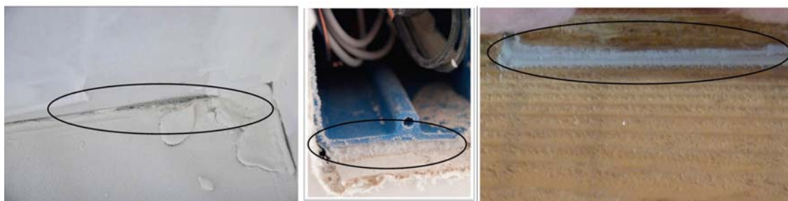
Figure 11. Photographs of envelope leaks sealed during the field tests (sill plate, electrical box, and header).
