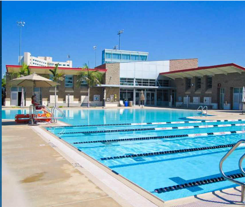
CATALYST RTU Efficiency Optimizer installed at San Diego State University's Aztec Aquaplex in San Diego, California
