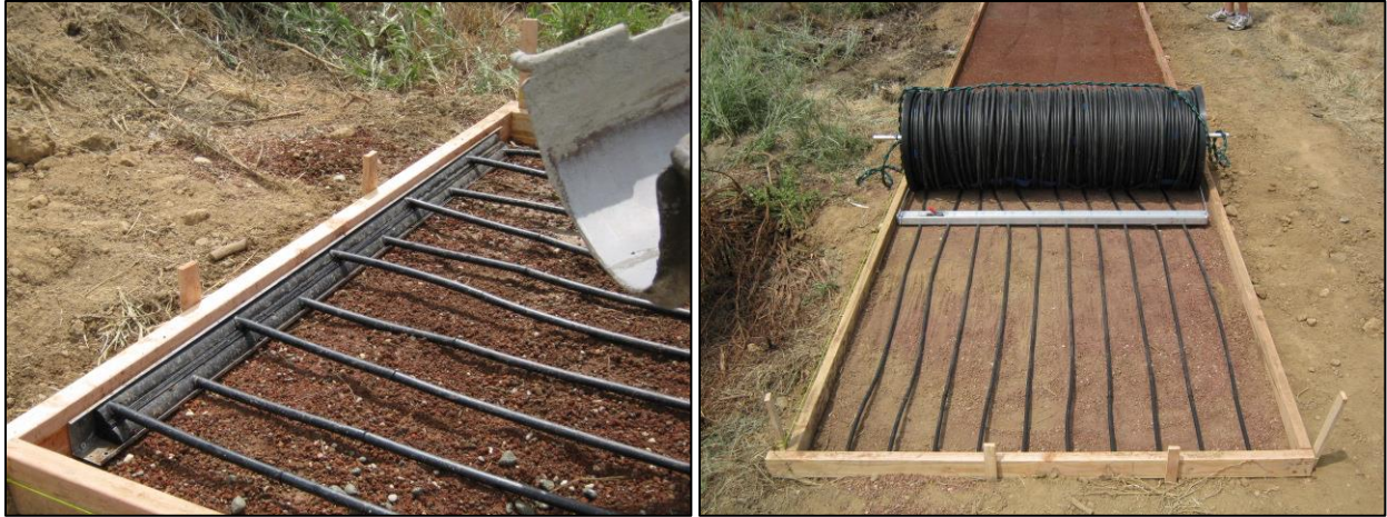
Figure 22 – Securing the manifold at the beginning of the installation (left) and setting up the spool and rake assembly for the rollout (right).
