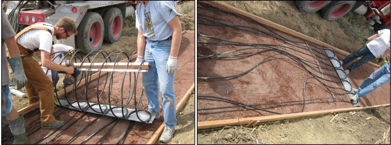
Figure 25 – Disassembling the spool to remove the spacer bars and end plate (left) and slack at the end of the roll in some circuits from imperfect rolling in the laboratory (right).
