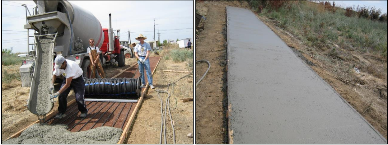
Figure 24 – Pouring concrete onto the tubes while moving the rake/spool assembly (left) and finished concrete (right).
