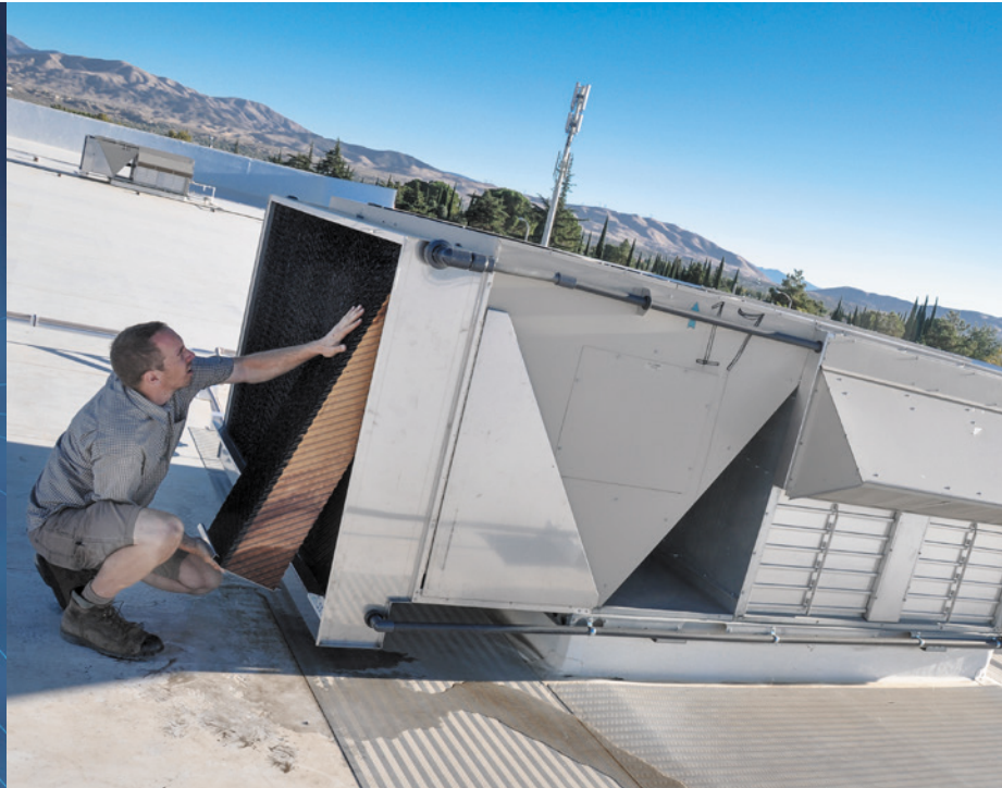
Dual evaporative pre-cooler installed in, Palmdale, CA
