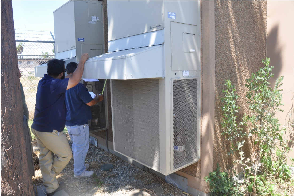
FIGURE 6: WALL PACK UNITS ON FIBERBOND STRUCTURE AT CUDAHY
