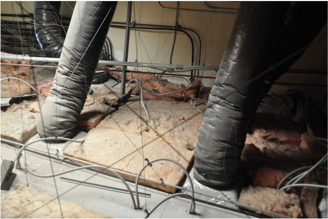
FIGURE 3: VIEW FROM ABOVE THE DROP CEILING OF CELL SITE ROOM AT PLACENTIA
