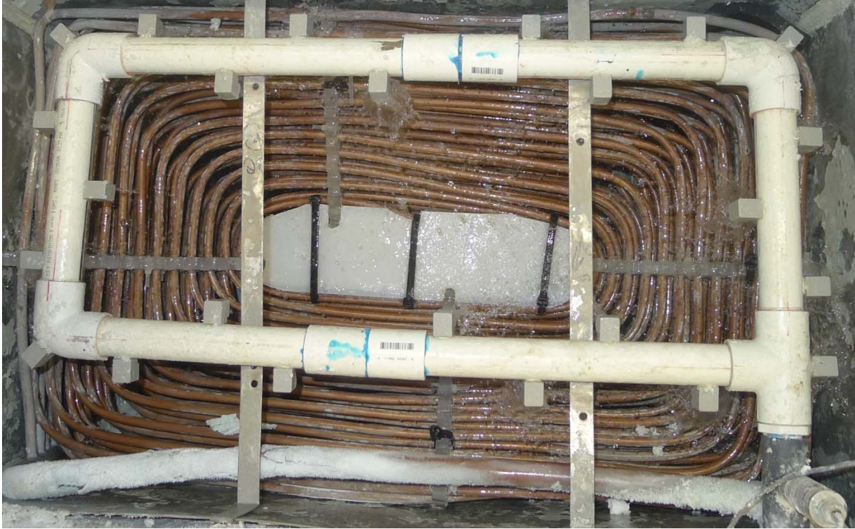
FIGURE 28. ECCU WITH LOW BLEED SPRAY PATTERN.
