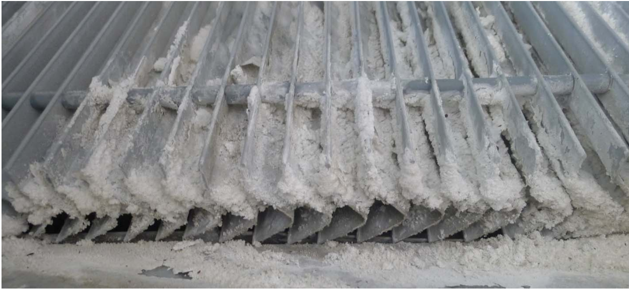
FIGURE 29. ECCU WITH LOW BLEED –SCALE FORMATION ON DRIFT ELIMINATOR
