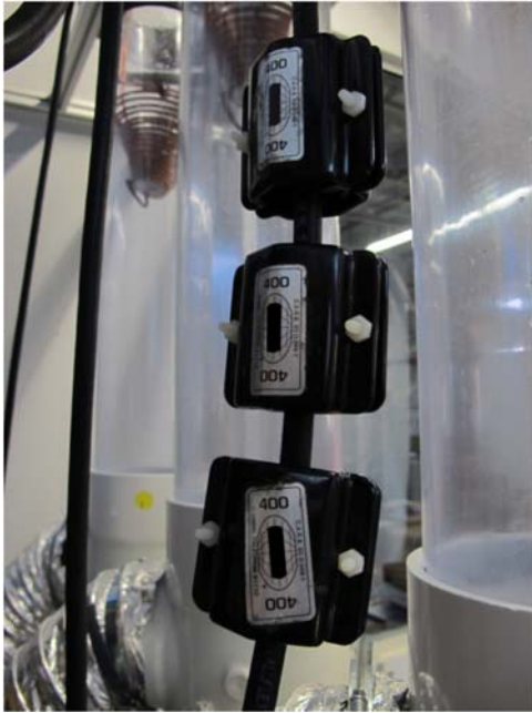
FIGURE 12. MAGNETIC TREATMENT ON COOLING WATER LINE
