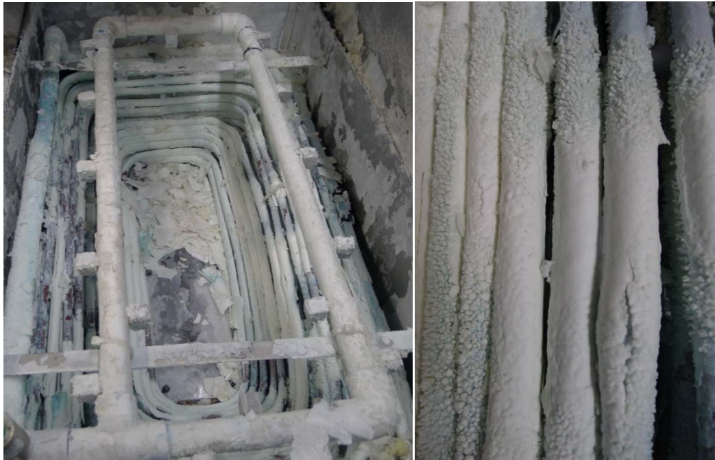
FIGURE 18. ECCU COOLING COIL FOULING. ENTIRE COIL (LEFT) MAGNIFIED SECTION (RIGHT)
