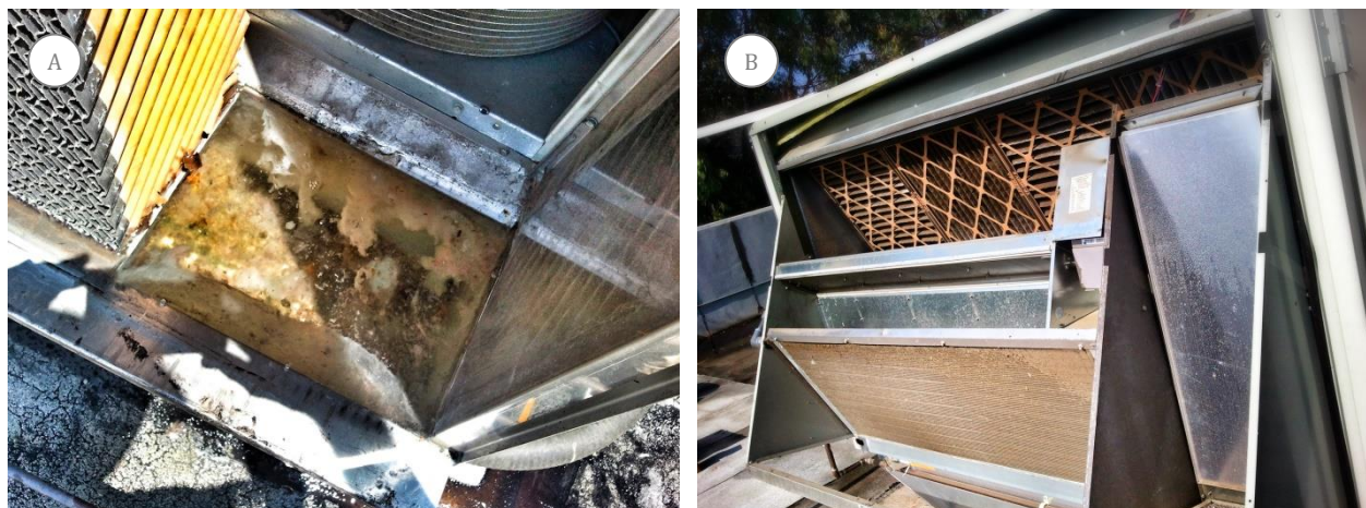
FIGURE 24: (A) BIOFILM ACCUMULATION IN SUMP (B) BUILDUP OF DIRT AND DEBRIS ON VENTILATION COIL
