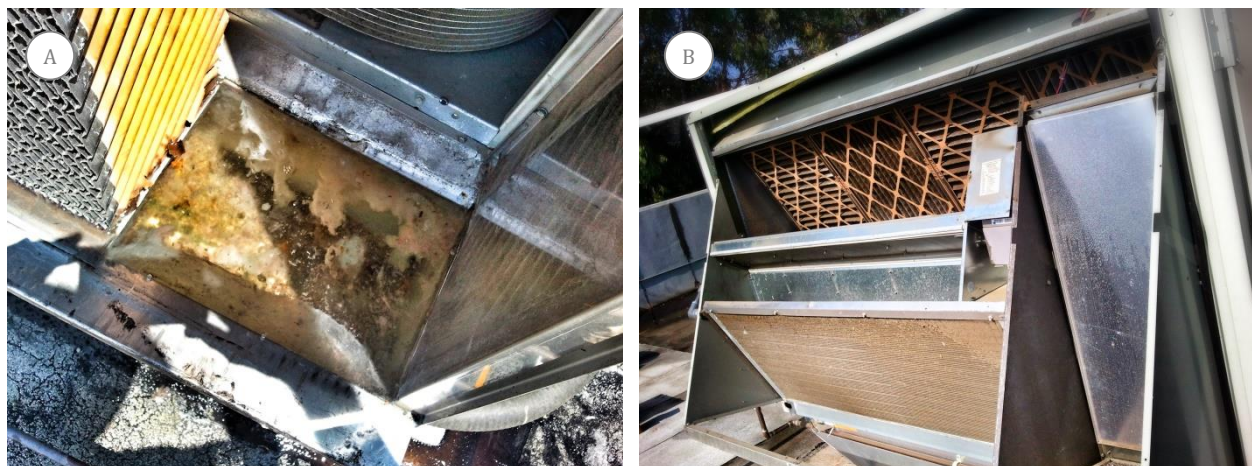
FIGURE 24: (A) BIOFILM ACCUMULATION IN SUMP (B) BUILDUP OF DIRT AND DEBRIS ON VENTILATION COIL
