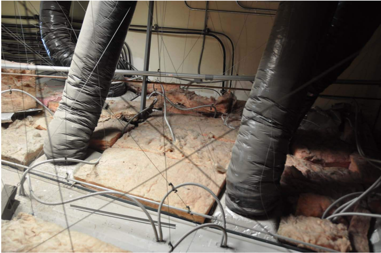
FIGURE 3. VIEW FROM ABOVE THE DROP CEILING OF CELL SITE ROOM AT PLACENTIA
