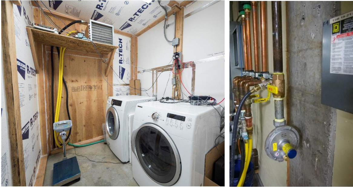
Figure 3 – Insulated wood frame chamber with heating, cooling, and dehumidification capabilities (left) and gas line and regulator (right).
