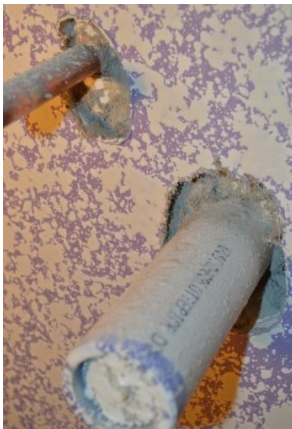
Water supply and waste pipes
