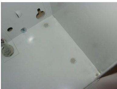
Kitchen fan housing interior
