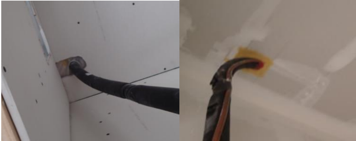
Figure 61: HVAC line set prior to any pre-sealing work (left) and after a manually applied permanent seal (right)
