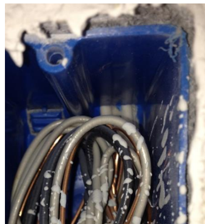
Electric outlet box
